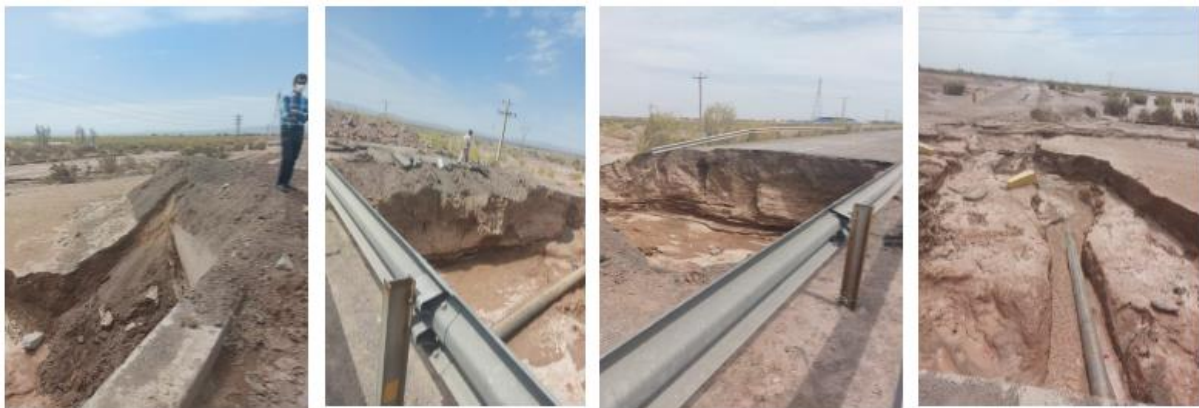
Fig 4. Field Visit on 05/01/1401 to the location of the damaged Rafsanjan-Sarcheshmeh road and the entry point of water into Jihad Town and Imam Ali boulevard (x=407352; y=3357783 UTM) - (Source: Authors)
