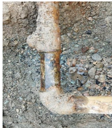
a) Crack damage in steel pipe
