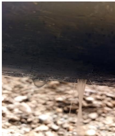
b) Hole damage in polyethylene pipe
