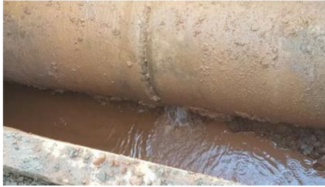
Figure 4. Sample Image (leakage at an incident location in water distribution network)
