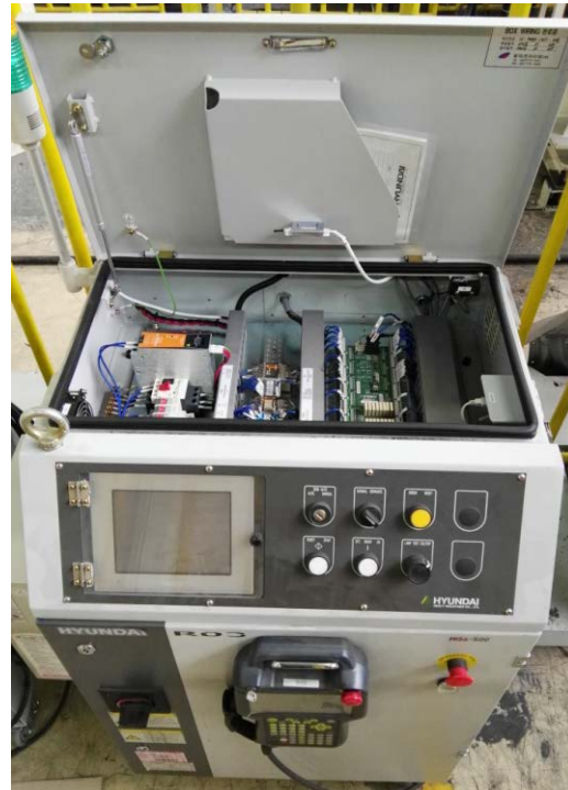
Fig.8. Embedded PLC section to interlock new generation robots
