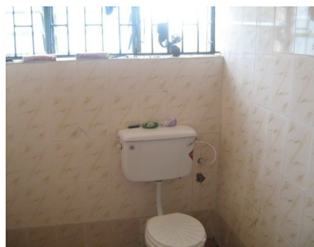
Fig.13: WC provided at UI hostel
