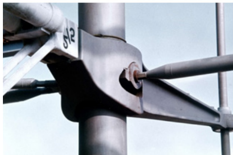
Fig. 11: The type of connections and joints used in the project of Georges Pompidou Center. France. 1977 (Source: Denancé & Berengo Gardin, 2017)
