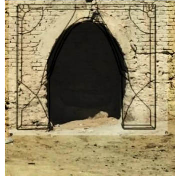
Fig. 51. Cracking pattern in QS-3
