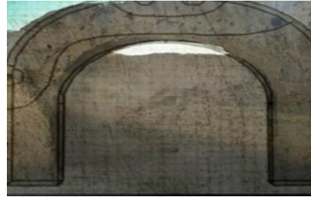
Fig. 41. Cracking pattern in QS-2
