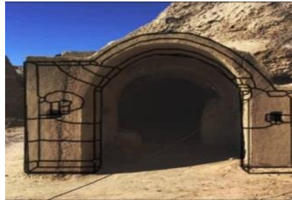
Fig. 31. Real-world example of the crack
