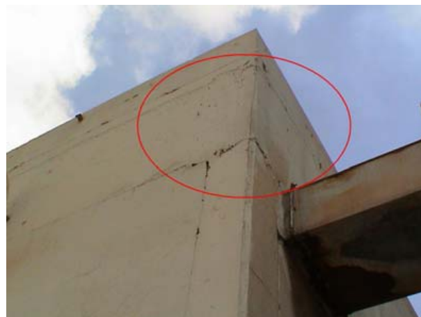
Figure 7. Strong beam, Weak column in both sides of structure
