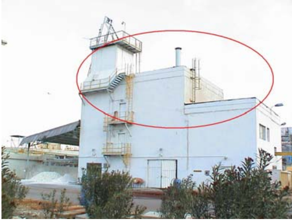
Figure 3. Photo of possible torsion condition
