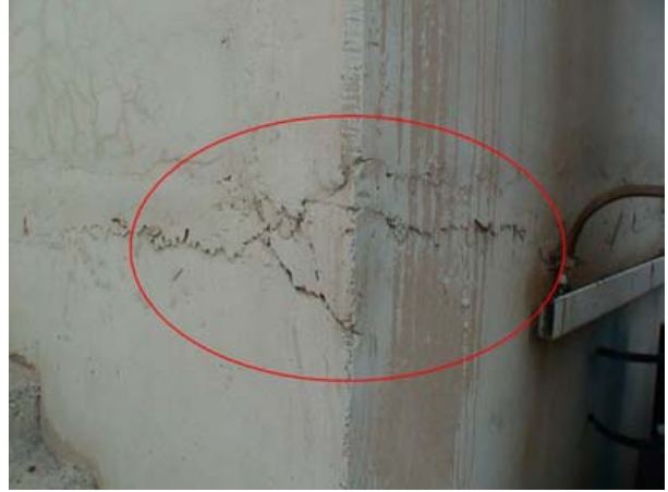
Figure 4. Cracks and degradation of R/C members
