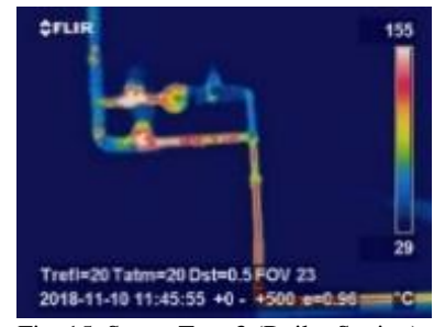
Fig. 15. Steam Trap 3 (Boiler Station)
