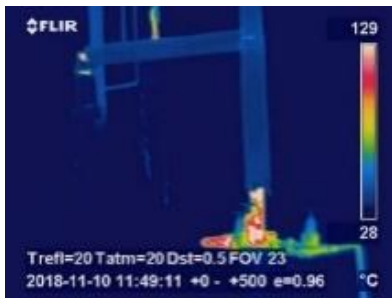
Fig. 13. Steam Trap 1 at Main Line Area (Boiler Station)
