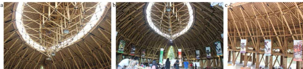
Fig. 10. OBI Great Hall structure system; (a) Skylight; (b) Trusses; (c) Details of braced frame [27].
