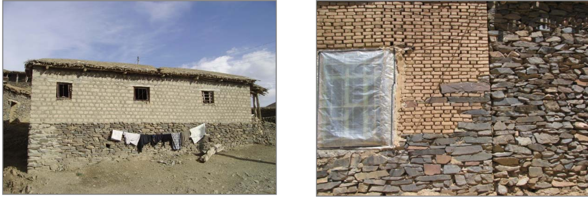
Figure (12): disharmonic materials such as bricks and cement blocks in the wall
