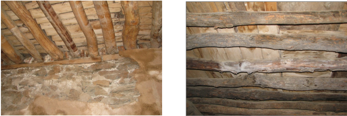
Figure (16): decay of ceiling wooden beams and interior wall plaster due to moisture permeability
