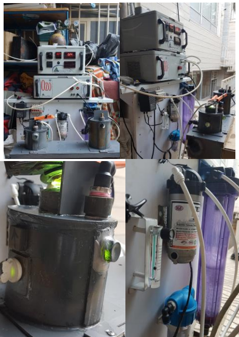
Fig 3. Ozone + UV pilot on the effluent of the coagulation process
