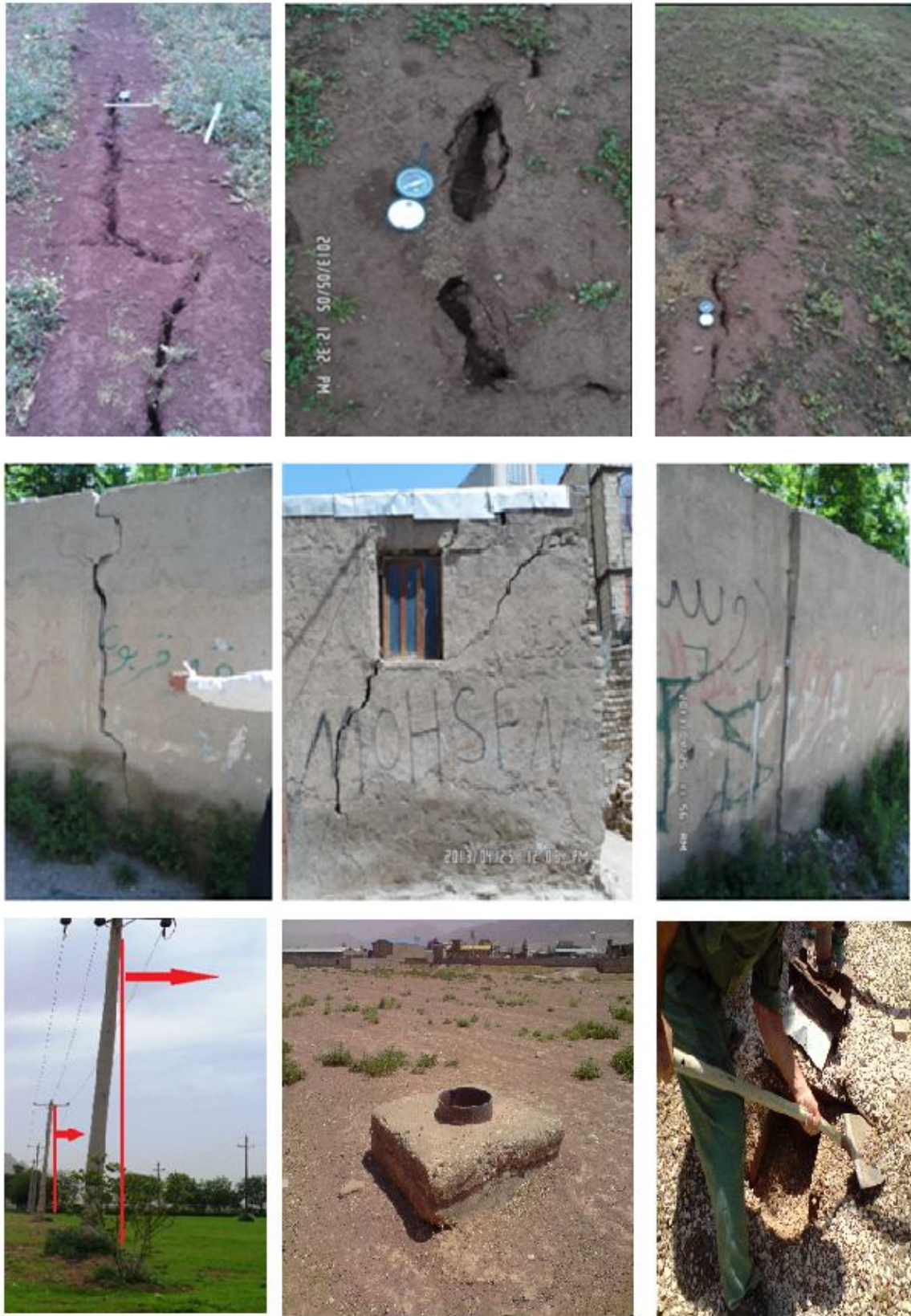
Figure 12. Evidence of subsidence due to increased effective stress of the drainage layers of the plain
