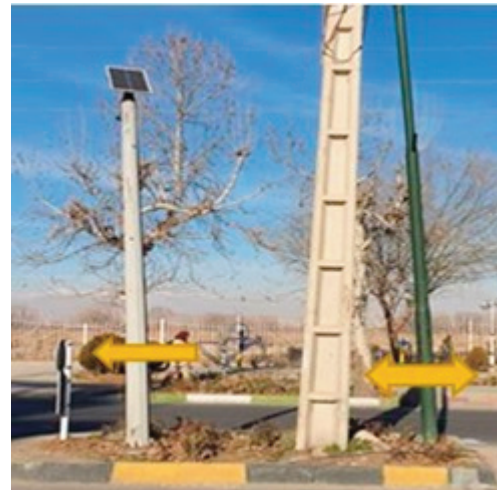
Fig. 6. Tilted electric post.
