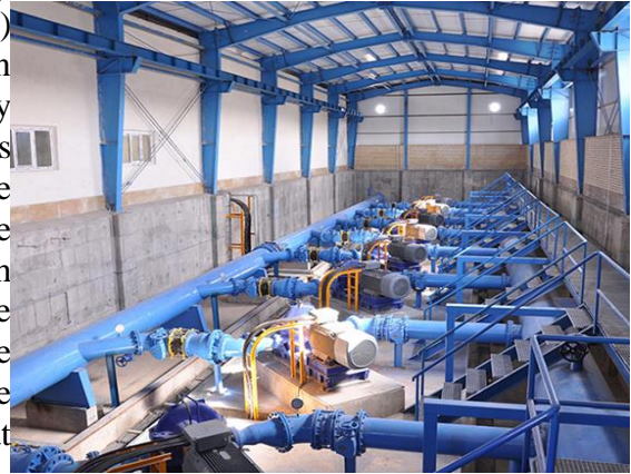
Figure 1. Pumping stations with horizontal pumps.
