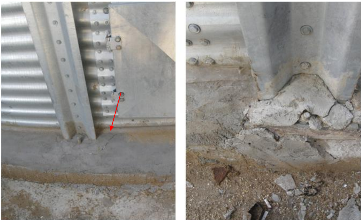
Figure 5. Detail of type "D" silos. Damage to foundation due to uplift of a bin
