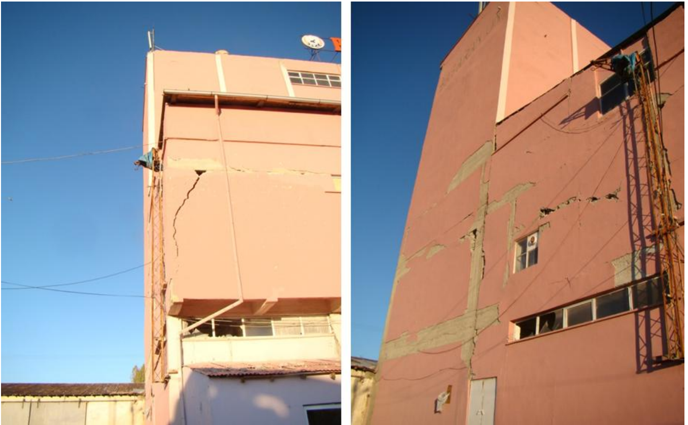
Figure 8. Out of plane failure of masonry infill walls of industrial buildings
