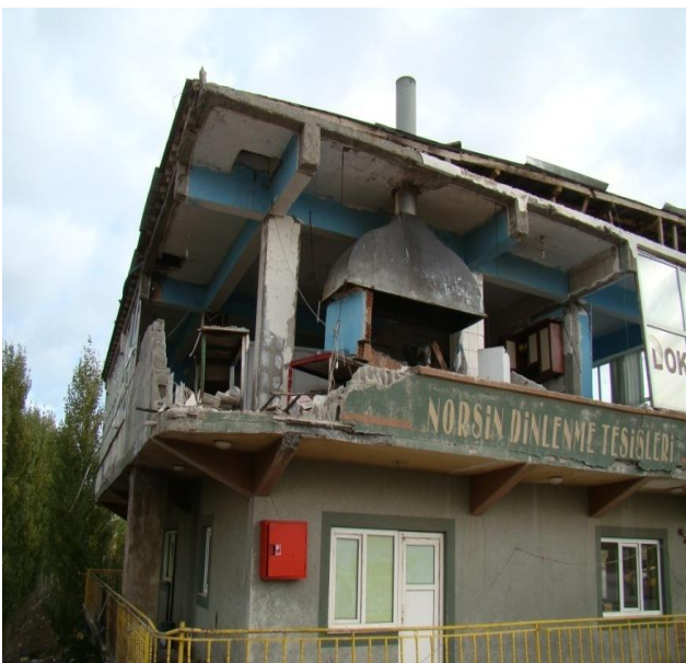
Figure 12. Noticeable damage to annex building of the gas station
