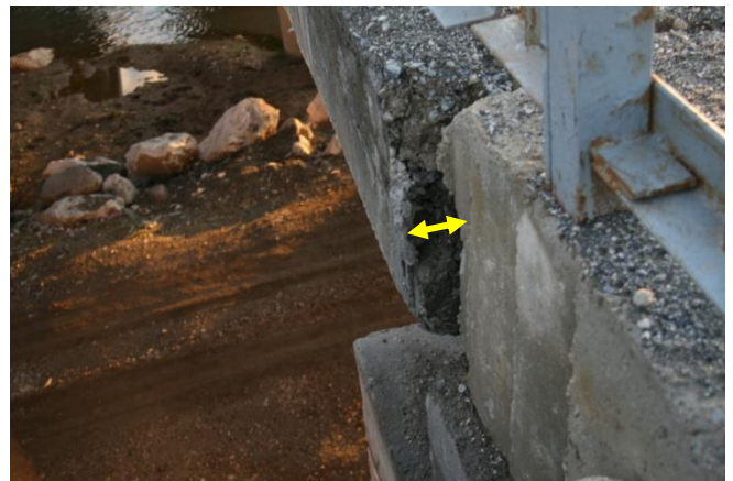
Figure 14. Damage to a RC bridge.
