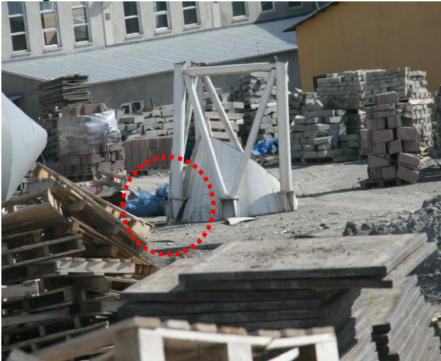
Figure 6. Failure of welds in shell to column connection of a cement silo
