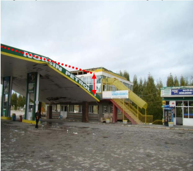
Figure 11. Collapse of the light weight roof of the gas station
