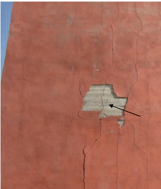
Figure 9. Observable crack in a RC wing walls in a low ductility RC industrial building.
