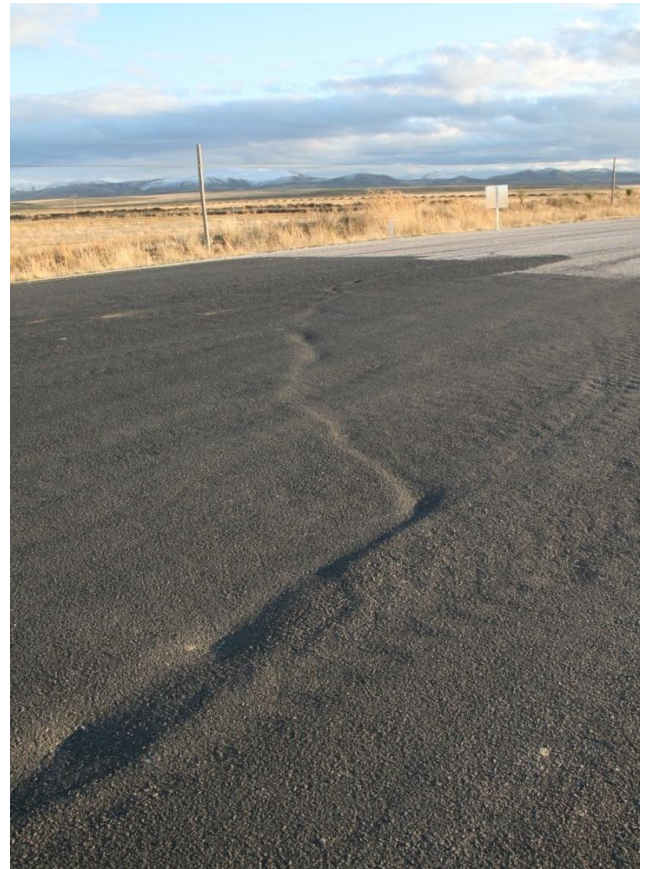
Figure 13. Cracks observed on road surfaces
