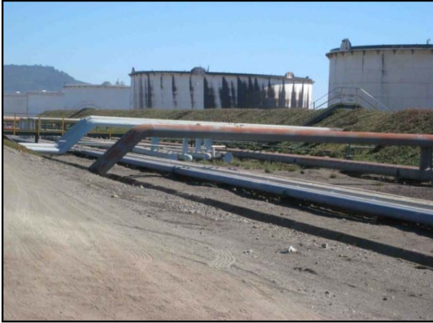
Fig. 22. Oil leak along the top edge of tank
