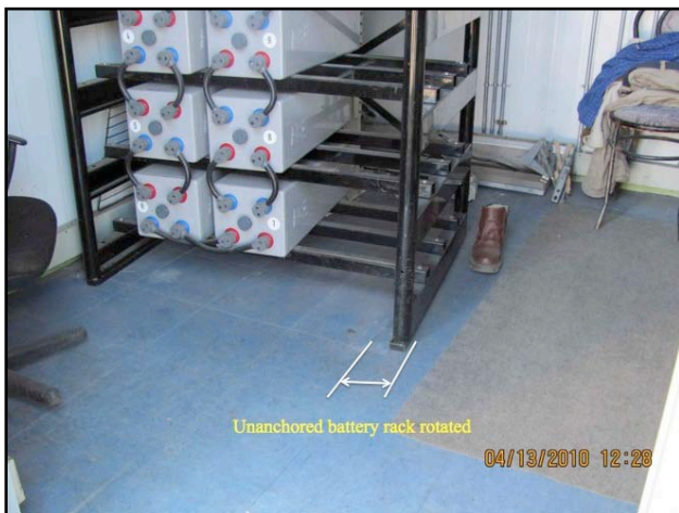
Fig. 5. Unanchored equipment in BTS
