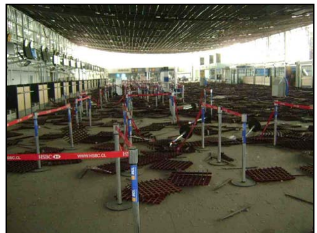
Fig. 11. Non-structural damage inside Santiago International Airport terminal (Public Works Chile photo)
