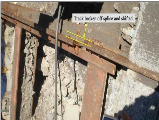
Fig. 9. Damage to railway track (Eidinger photo)
