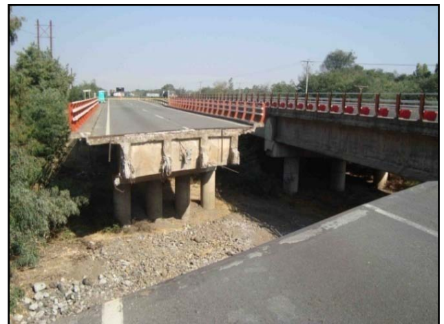
Fig. 7. Hwy #5 bridge collapse, south of Linares
