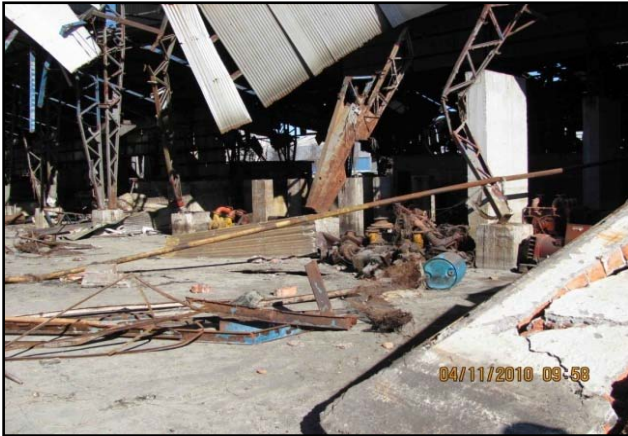
Fig. 16. Fish processing plant damaged by tsunami
