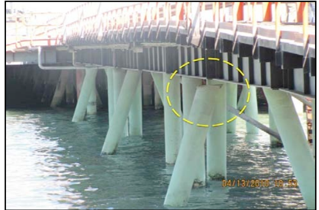
Fig. 18. Coronel Port pier #1 - pile with weld broken off
