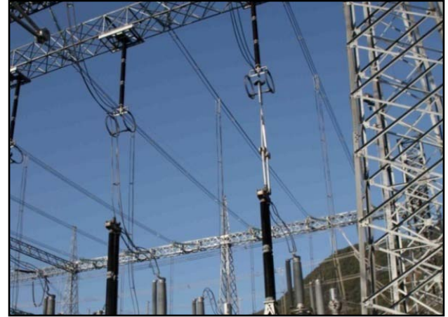
Fig. 2. Candlestick style disconnect switch (Kwasinki photo)
