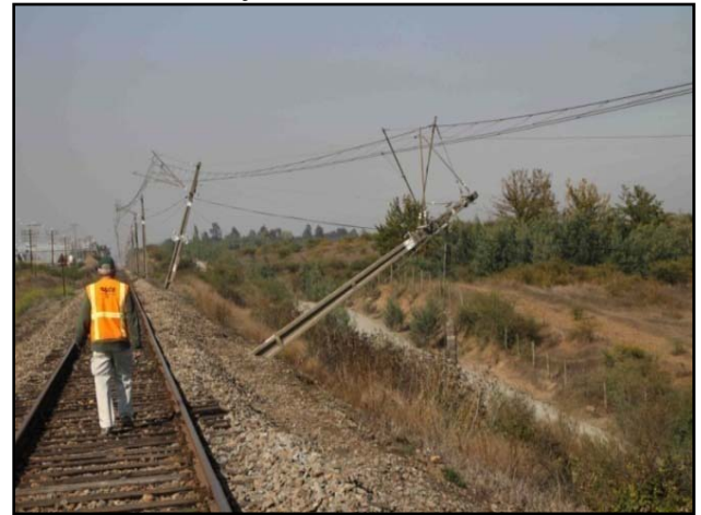
Fig. 10. Damage to power poles for railway trains (Eidinger photo)
