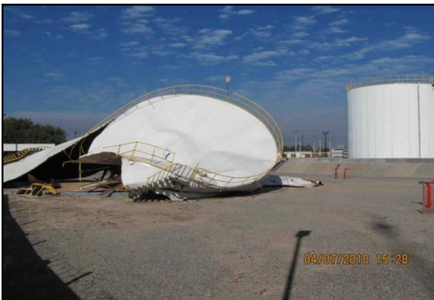
Fig. 23. Water tank for fire fighting – Santiago International Airport
