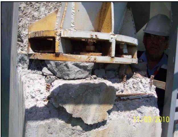
Fig. 13. Control tower cabin anchor points damaged due to short edge distance
