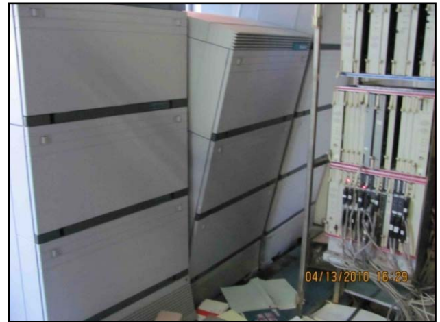
Fig. 4. Switching equipment damaged in a CO in Concepción
