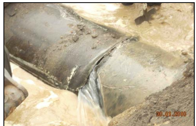
Fig. 24. Broken steel water pipe (Essbio)
