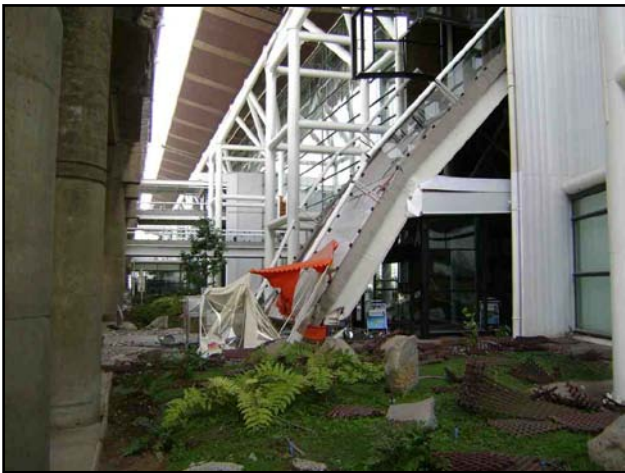
Fig. 12. Damage of overpass connected between the terminal and the raised access road (Public Works Chile photo)
