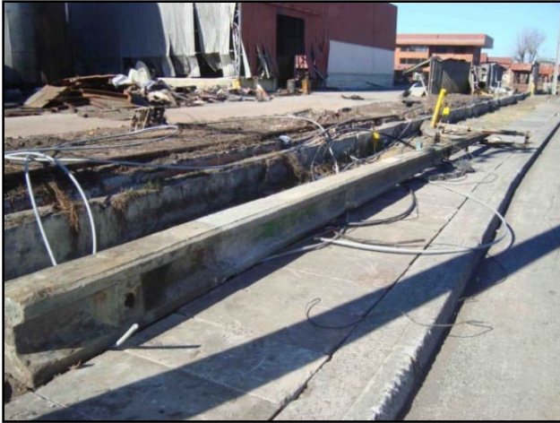
Fig. 3. Typical power distribution system damage
