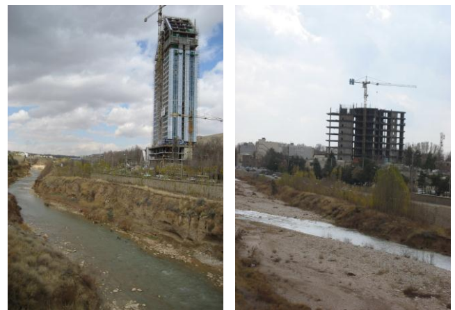
Fig. 2, 3. Effects of construction on the river landscape
