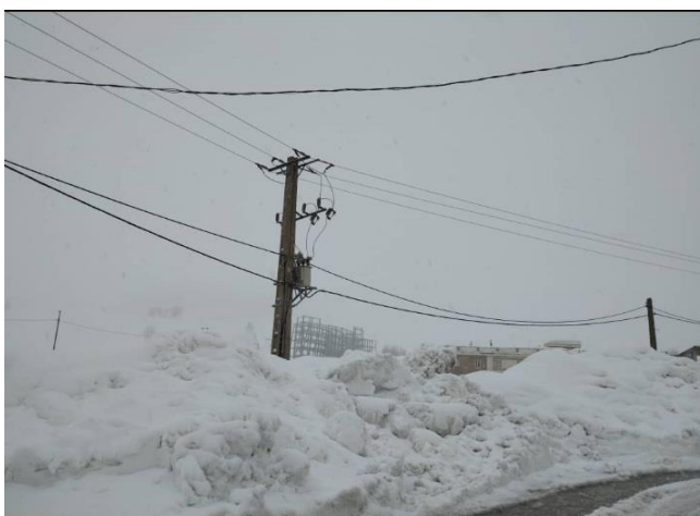
Fig.14: The distribution board falling under the snow
