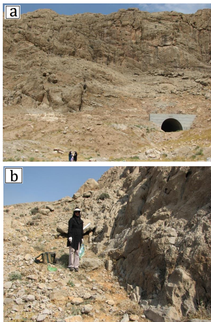
Fig 12. a) Train tunnel through rock making thick- bedded to massive limestones of Sarvak Formation, b) Contact between Sarvak and Ilam Formations as a depositional disconformity.
