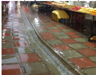
Fig9: Drainage gradient for disposing the surface water of the pathways in Asef Bazaar
