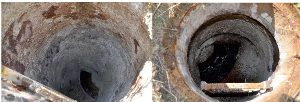
Fig. 1. Typical damage of concrete elements caused by MICC in different sewage systems (Grenng et al., 2018).
