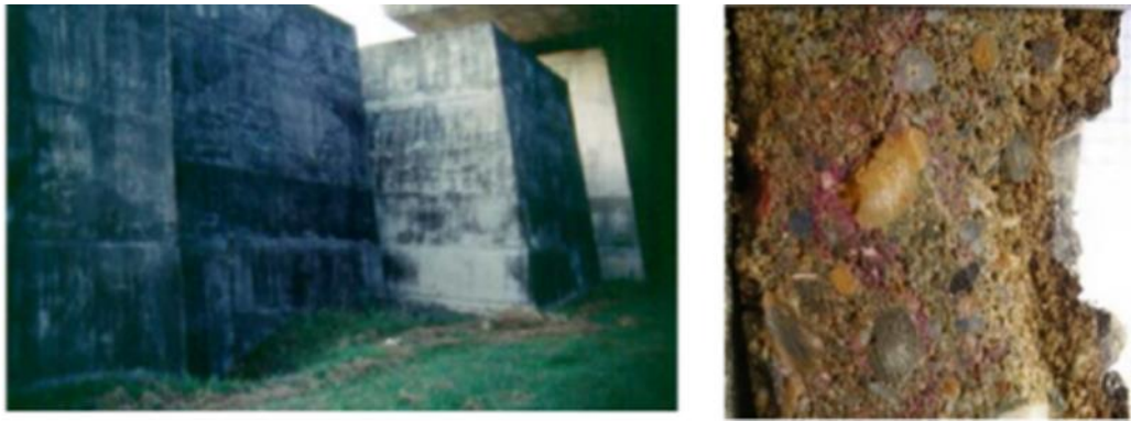
Fig. 2. cases of biological degradation of concrete (Jiang et al., 2022).
