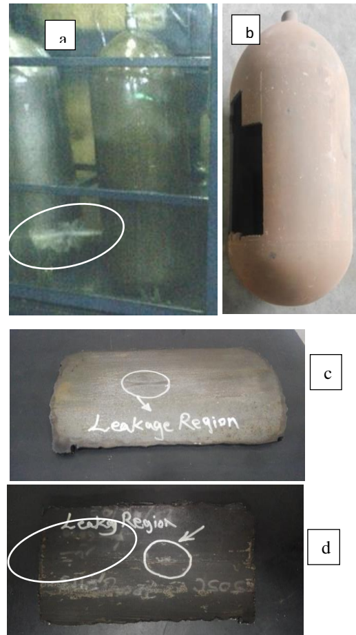
Fig. 11 (a): cylinder is leaking from the cylindrical part under test, (b): the leakage area is cut out to internal and external inspection, (c): external surface of leakage area, (d) internal surface of leakage area
