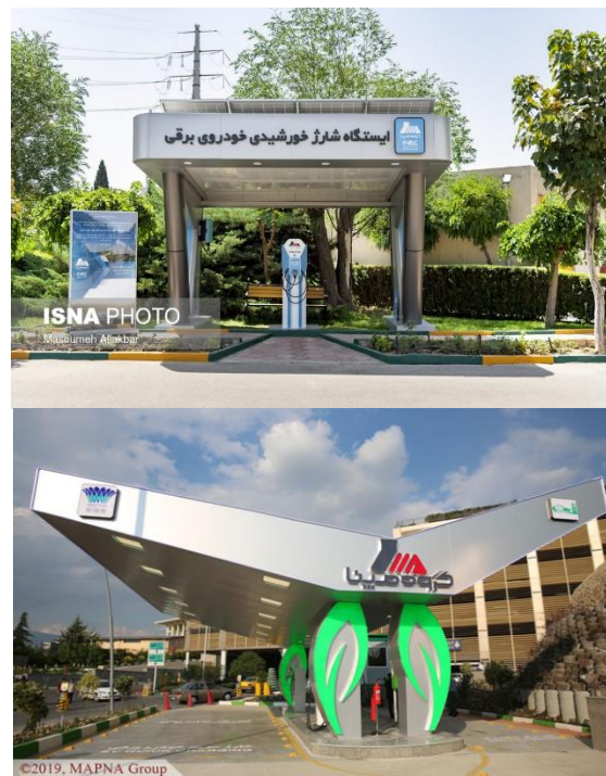
Fig. 3. The first EV charging station in Iran and the first solar EV charging station in Alborz province
