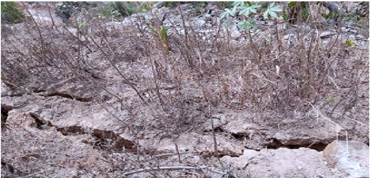
Figure 2. A view of tension cracks on the ALUT landslide
