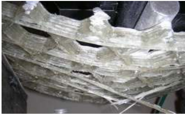
Fig. 7 Failure in bottom layers.
