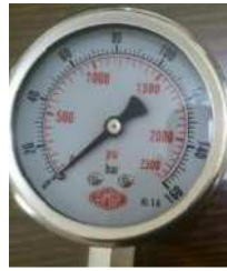
Figure19. Pressure gauge installed on system
