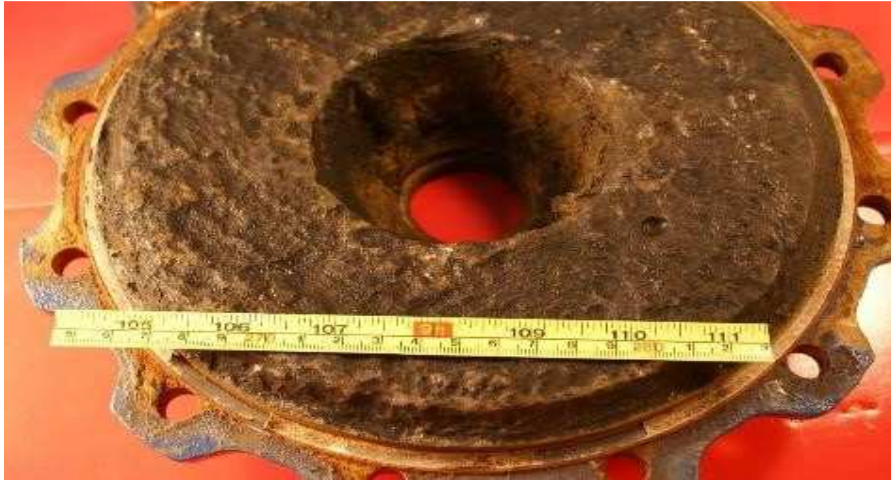
Figure5. Damage and the formation of deposits on the inner cover of the pump
