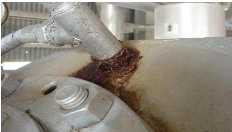
Figure7. Corrosion at the junction of cooling water system to the compressor
