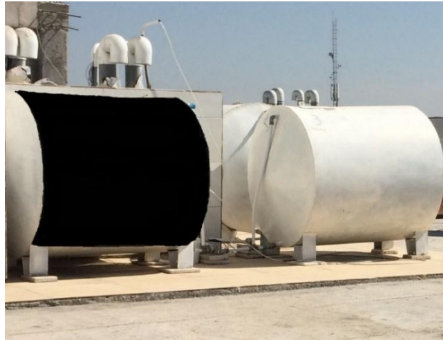
Fig. 10. Dark and white water tanks on the roof
