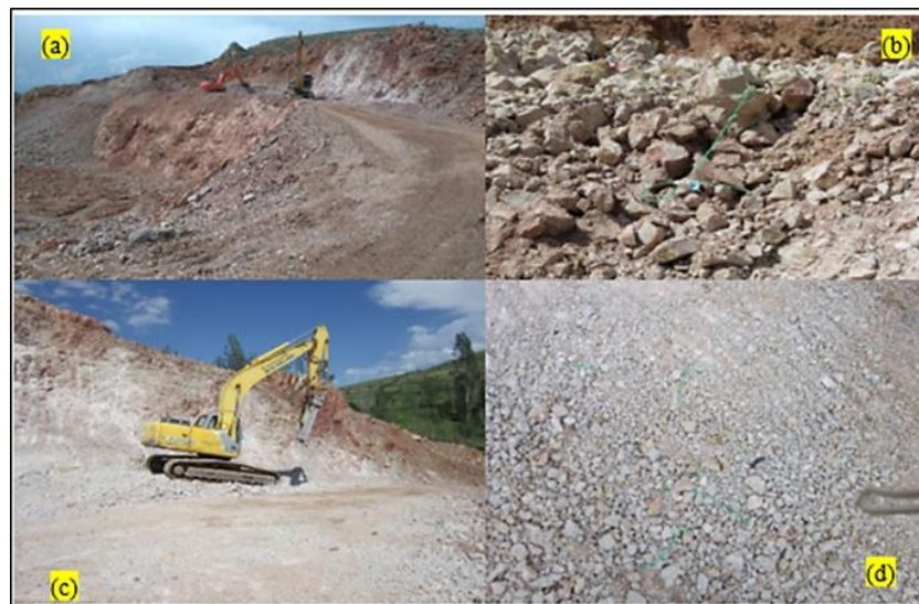
Fig 11. Excavation method currently applied at the study site and equipment used. (a) drilling holes for pre-excitation loosening blasting, (b) loosening blast, (c) excavation and size reduction with hydraulic breaker, (d) final product state
