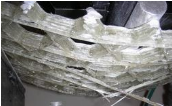
Fig. 7 Failure in bottom layers.
