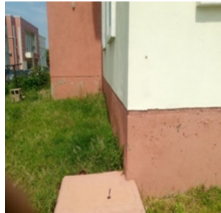
Fig. 12: Painting on the wall of the building peeling off.
