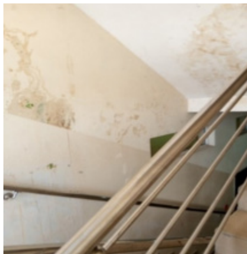
Fig. 13: Traces of Spirogyra and dampness noticed on the wall and underneath the staircase due to poor position or maintenance of the water reservoir
