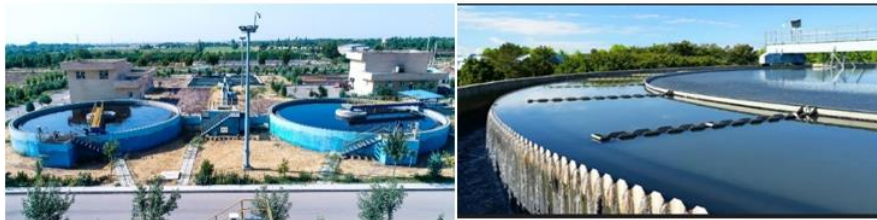
Figure 2: Output of the MLE Wastewater Treatment Plant in Mahmoudabad, Qazvin.
