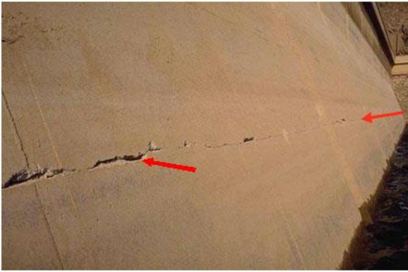
Fig.11. Downstream cracks view of rib number 18
