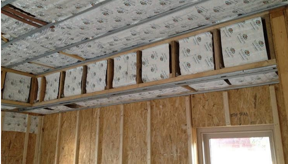
Fig 7- Use of phase change materials in the interior walls of the building
